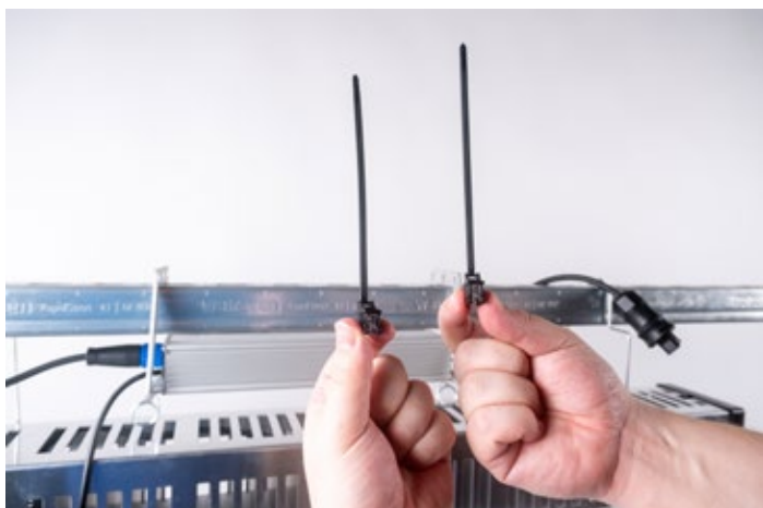
Step 9: Get the cable binders.
